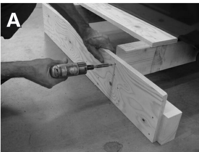
Remove the screws from the board on the front side of the pallet as shown above
